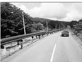
Fig.5 Pipeline from production station to power station
